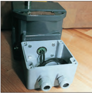
Line bushings in the Ex e terminal box
